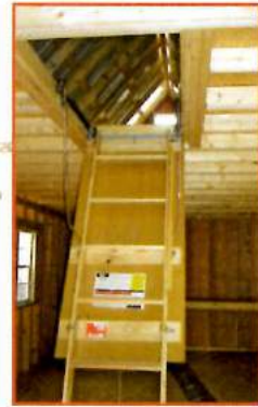
PULL DOWN STAIRWAY
